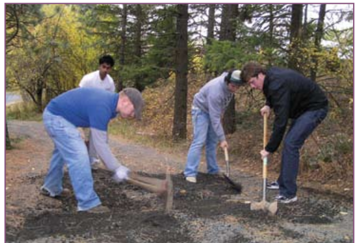
Students from UI CORE discovery course repairing the parking area at Idlers Rest
